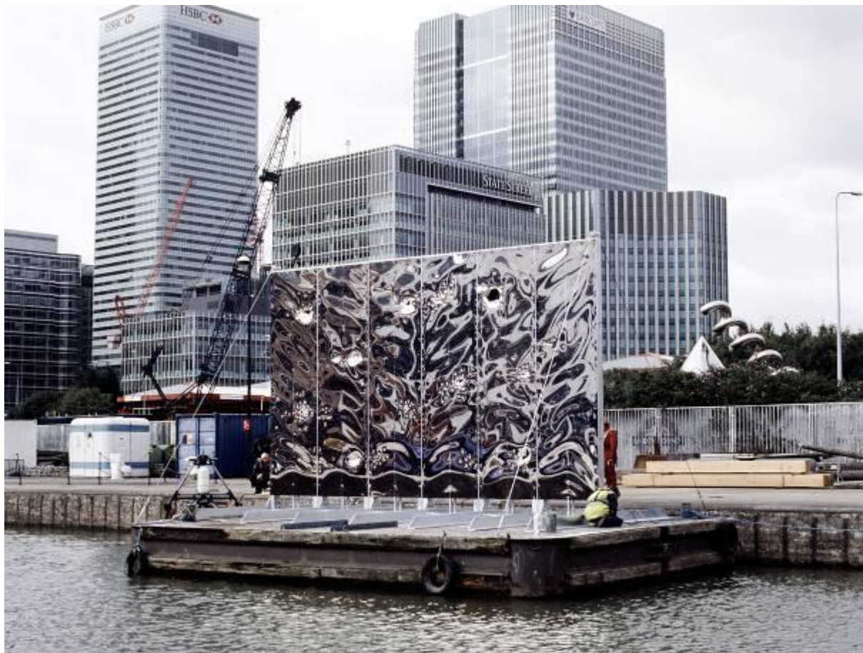
Installing at Canary Wharf dock – 'Saved from Drowning'. 2008 Mirror polished steel, galvenised steel, tension ropes, steel bolts.
